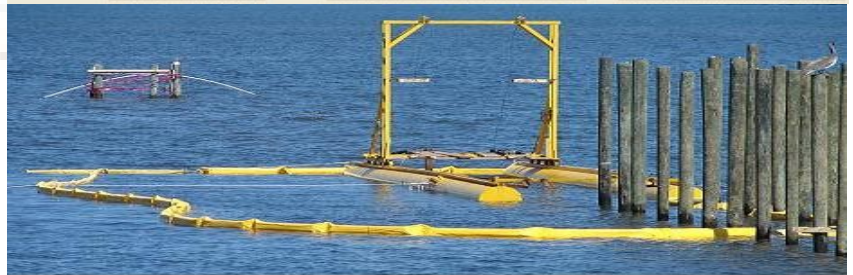
Type 1 Silt Barrier used on a pile driving on Intercoastal - Florida USA
